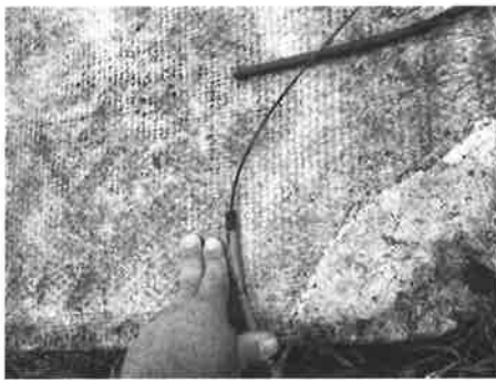
24 strand cable inside Micro Duct
